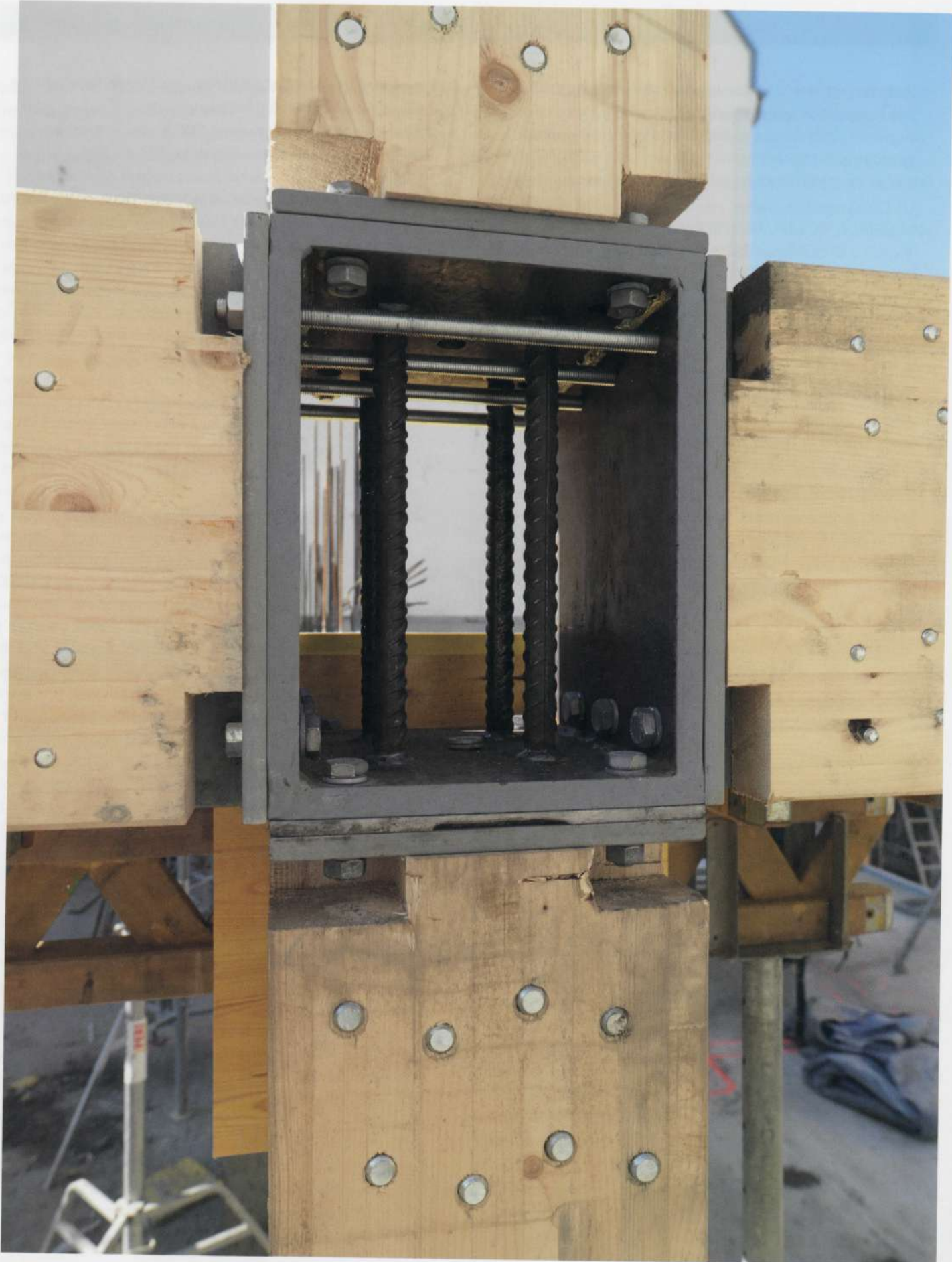
4.1.1 Detail of timber connection at forthcoming concrete beam. See e_3 case study for more information. Source: Kaden + Partner Architekten
