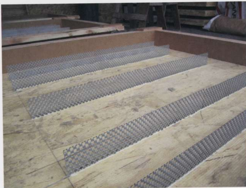
3.1.14 Steel mesh epoxied into CLT floor panels before pouring concrete slab. Source: Structurlam
