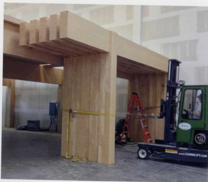
3.1.4 LVL columns, beams and floor components during construction. Source: Brisco Manufacturing Ltd.
