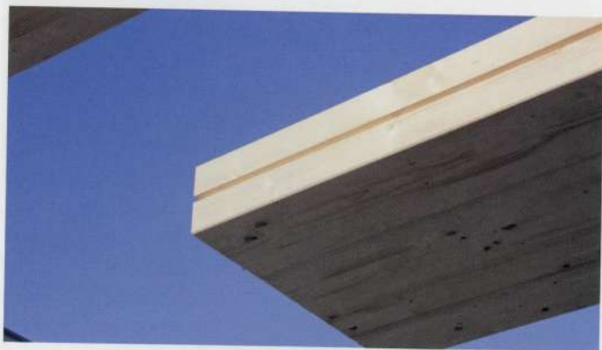
3.1.3 Glue-laminated timber panel during construction of Kuchl Campus Extension Building. See case study for more information on project. Source: Salzburg University of Applied Sciences
