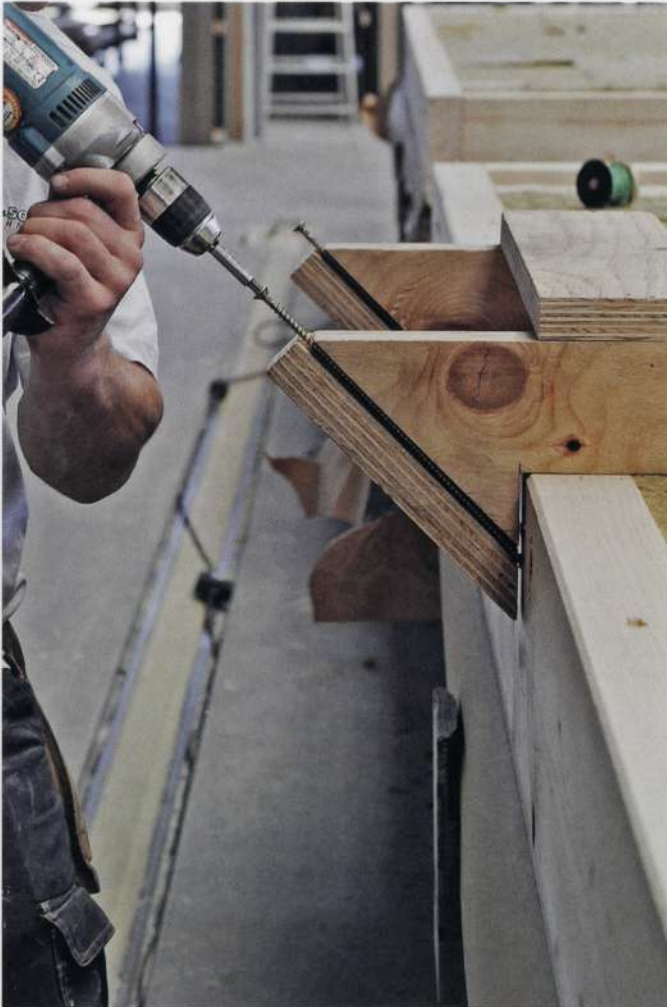
3.1.18 Prefabrication of solid wood wall panels. See H8 case study for more information. Source: Huber & Sohn
