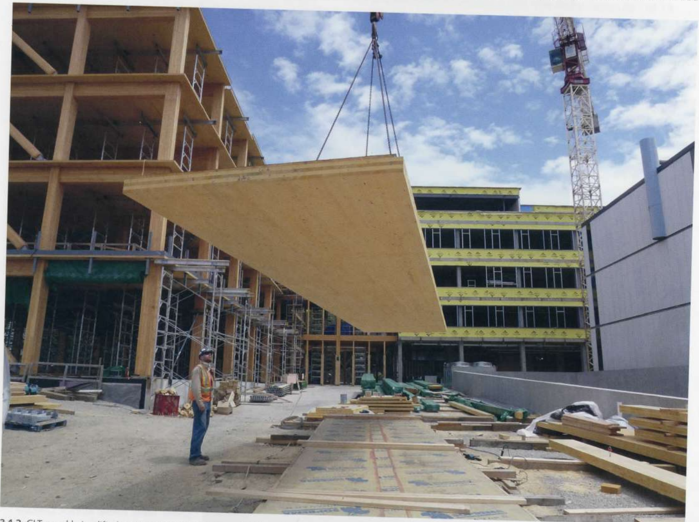
3.1.2 CLT panel being lifted into place at Earth Sciences Building (ESB). See case study for more information. Source: Structurlam
