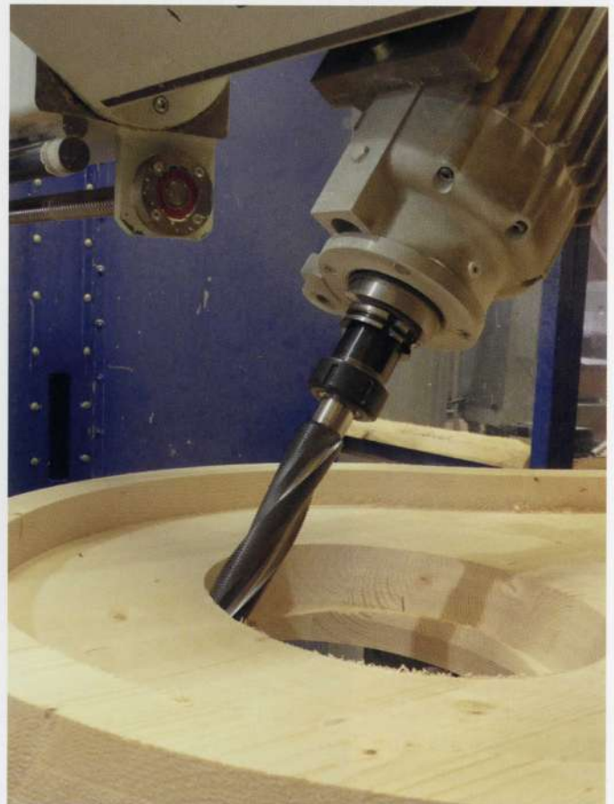
3.1.15 CNC fabricating wood building component. See Tamedia case study for more information. Source: Blumer Lehmann AG
