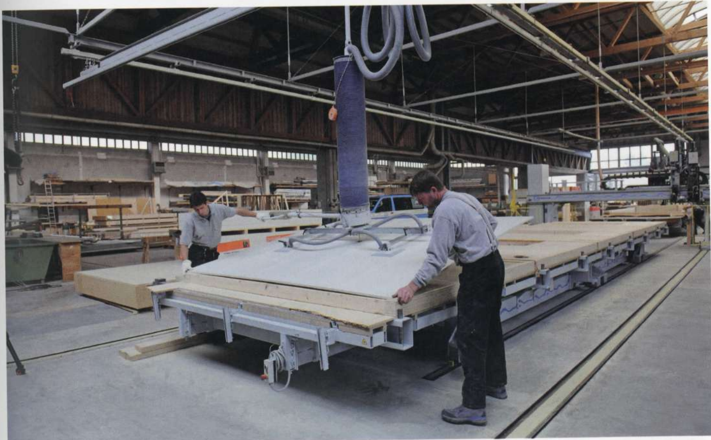
3.1.20 Installing gypsum board cladding to prefabricated wall in the factory. Source: Huber & Sohn
