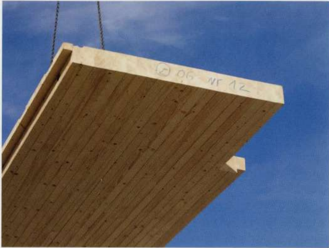
3.1.10 Dowel laminated panel being lifted into place. For more information see e_3 case study. Source: Kaden + Partner Architekten
