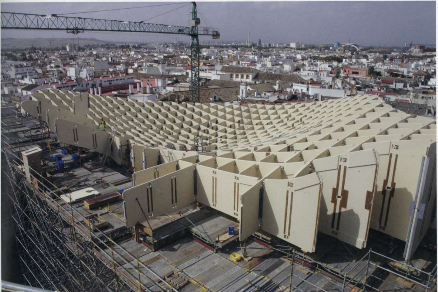
3.1.17 The Metropol Parasol in Seville, Spain during construction. Source: Jan-Peter Koppitz, Associate at Arup
