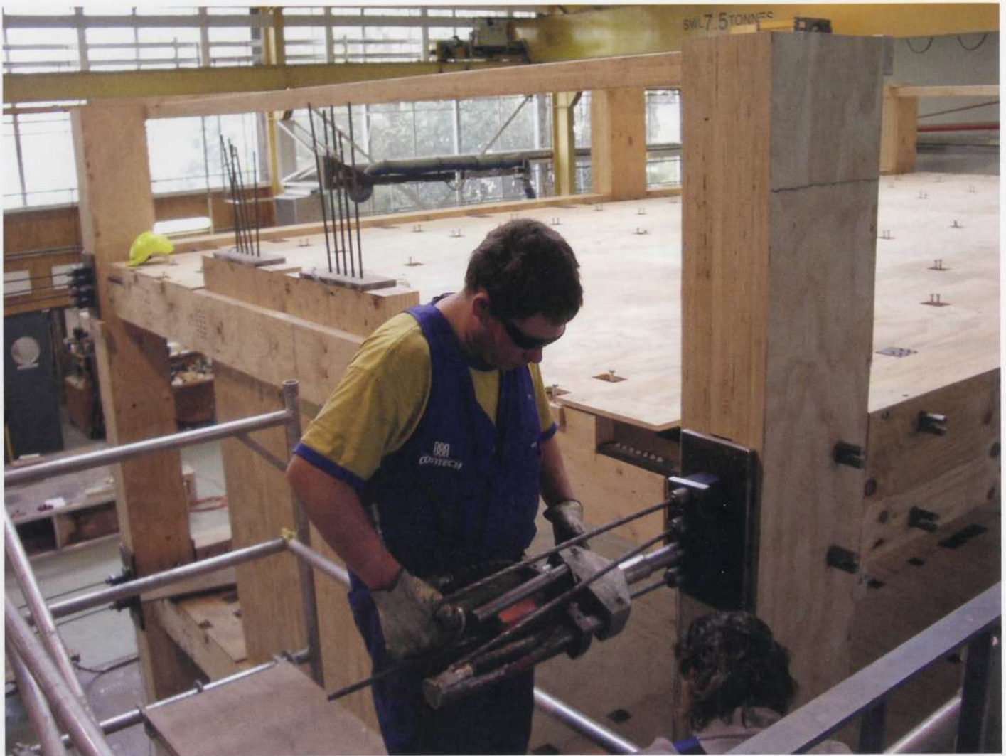
3.1.12 Tensioning steel cables in post-tensioned timber frame. Source: Professor Andy Buchanan, University of Canterbury
